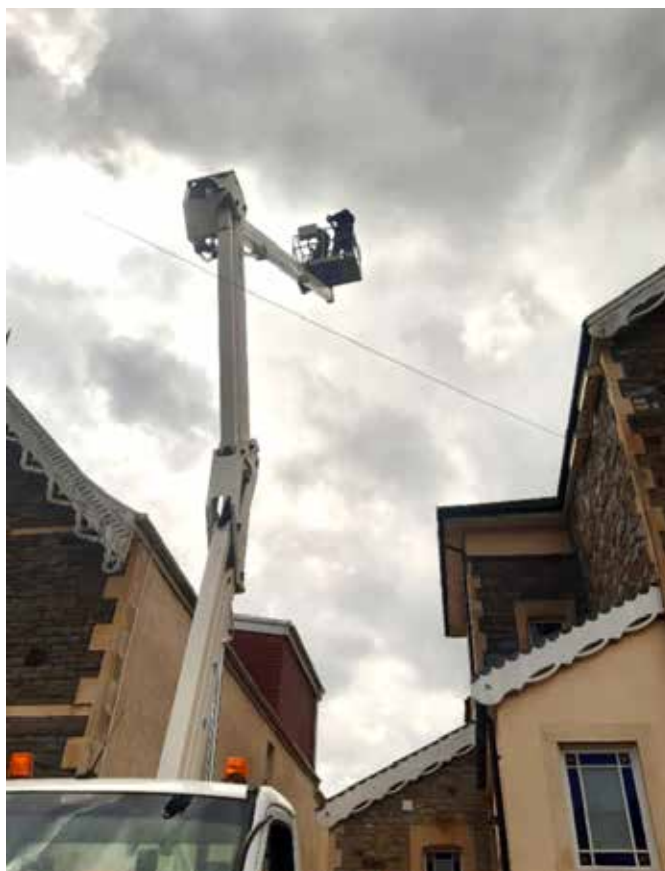
Two double boxes just installed on the house on the right. Toby and Justin decide to check the swift's eye view, which you can see below
